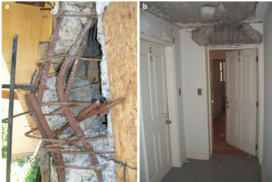
Fig. 39.9 (a) Buckling in longitudinal reinforcement bars first floor columns. (b) Lintel beam cracked
